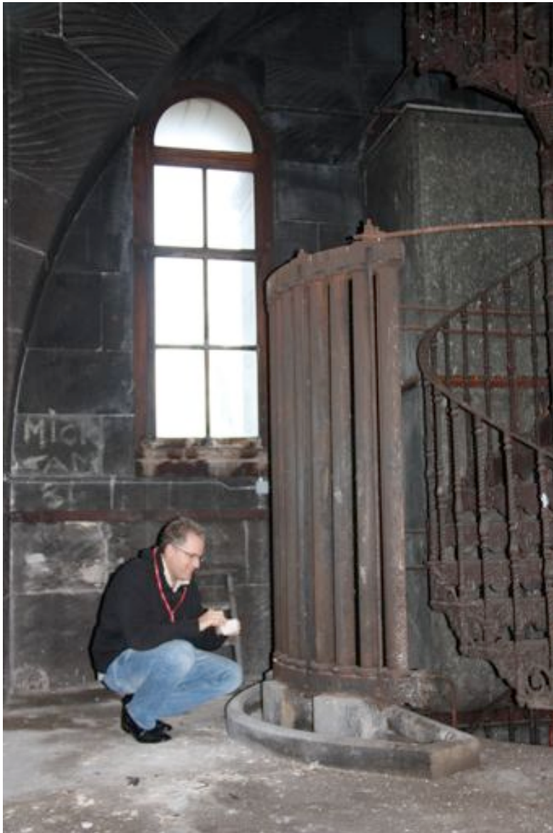
Ken Horrigan inspecting components of an early heating and ventilation system at Glasgow City Chambers
